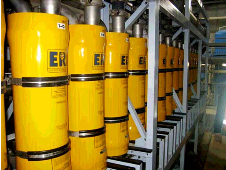
Figure 6-24 ERI PX energy recovery device at Perth's Kwinana SWRO
