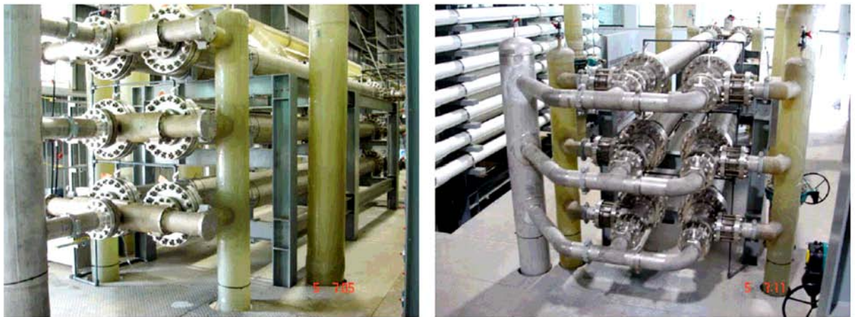
Figure 6-25 Completed Triple DWEER Energy Recovery systems at the Singapore desalination plant, April 2005 8
