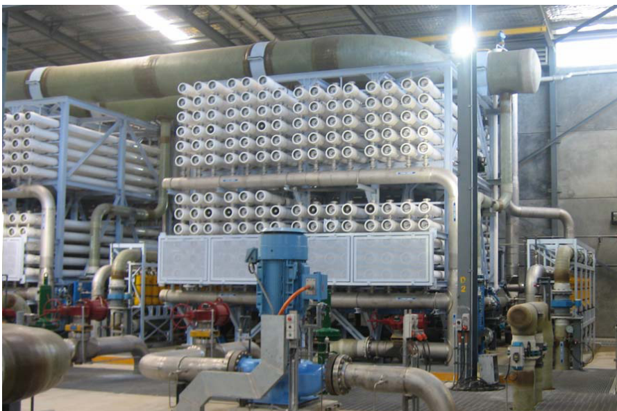
Figure 6-20 Rack of RO pressure vessels, Perth Desalination Plant 7
