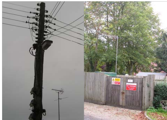
Fig 55, Unightly wirescape Poor landscaping around electricity sub-station
