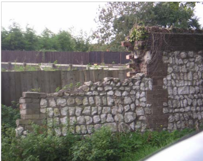
Fig 54, Eroding historic wall which has been repaired with inappropriate concrete mortar.
