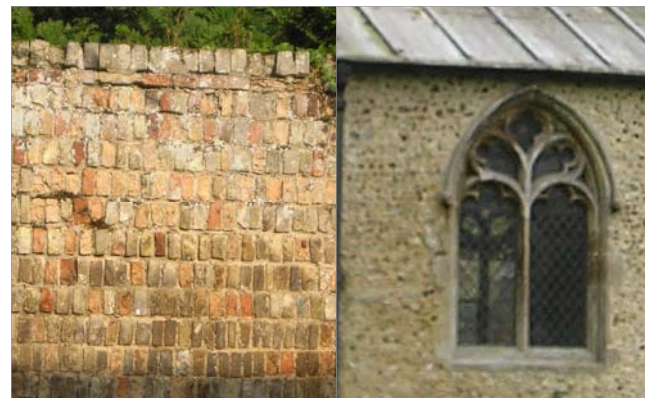
Fig 45, Local red brick laid on edge Fig 47, Flint, stone & lead on the St. Mary's Church
