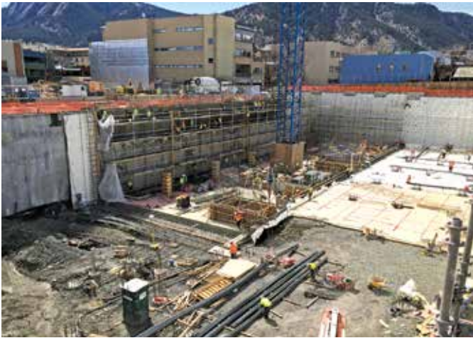
Figure 13. View of the preapplied sheet waterproofing being installed over the support of an excavation wall at a zero-lot-line condition.
