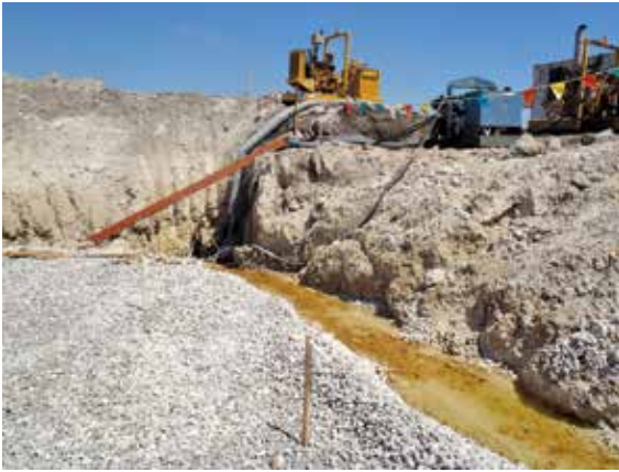
Figure 8. A dewatering pump station at a perimeter trench at the corner of the building pad.
