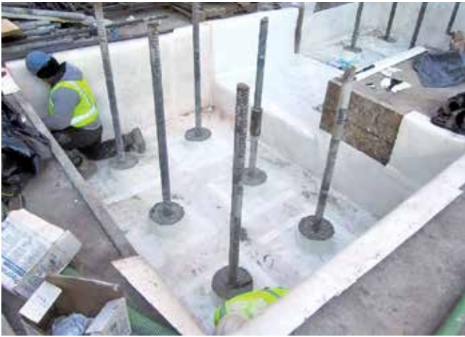
Figure 3. Rock anchor penetrations through foundation waterproofing.
