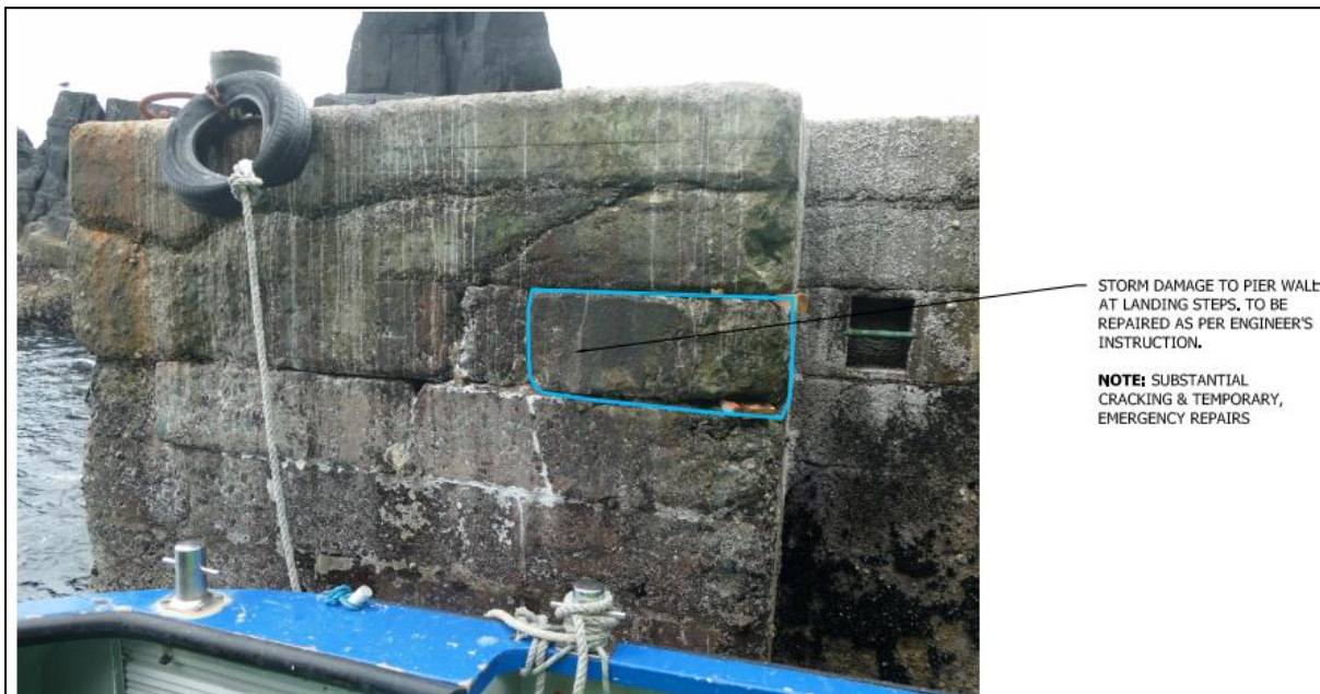
Figure 8. Storm-damaged block work in pier wall
