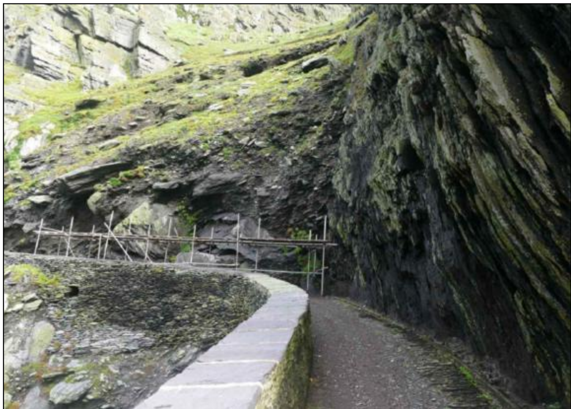
Plate 4. Temporary crash deck installed at location of proposed crash deck 3 on the Upper Lighthouse Road
