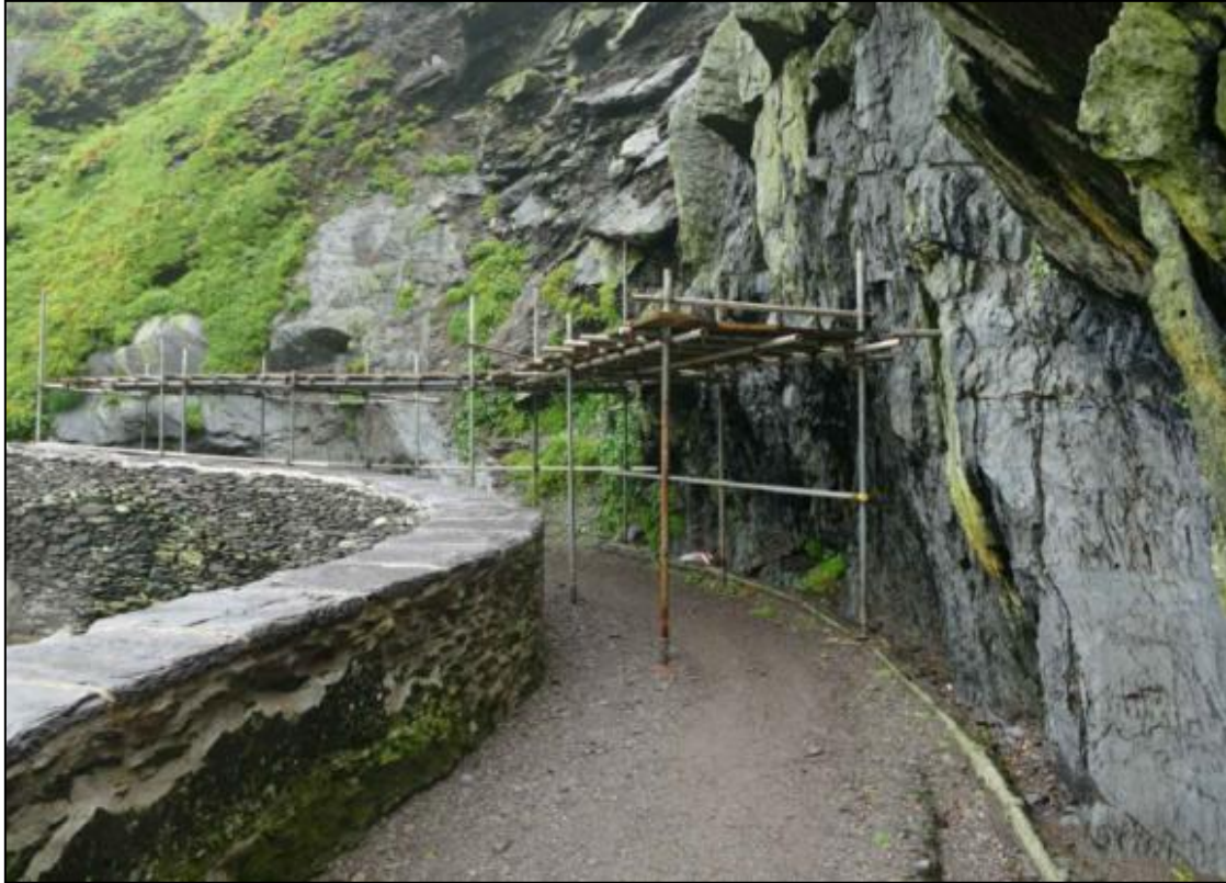
Plate 3. Temporary crash deck installed at location of proposed crash deck 2 on the Upper Lighthouse Road
