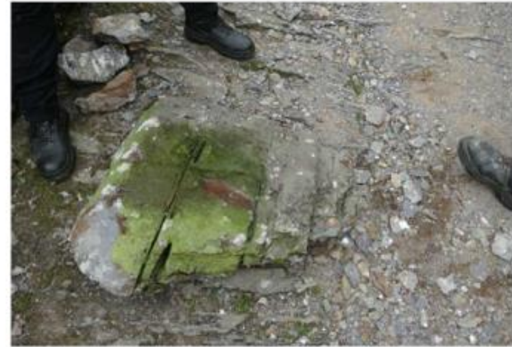
02 007 View of existing rock from the rock fall that occurred on 13.06.2022
