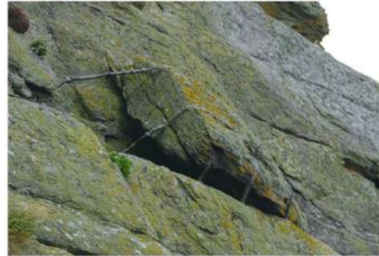
04 007 View of existing rock held in place by metal straps above lower lighthouse road
