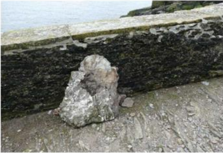
01 007 View of existing rock from the rock fall that occurred on 13.06.2022
