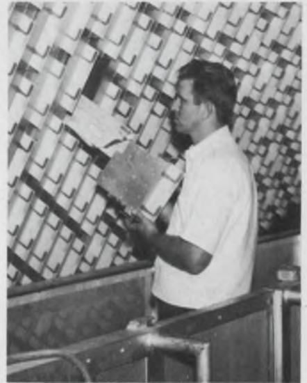
A phase-shifter module is installed in the collecting side of the large microwave lens in the new radar.
