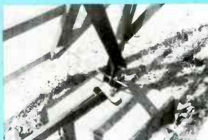
FIG. 26—CONCRETE BASE PADS support and anchor the four corners of the antenna. Anchor bolts and "J" clips secure the antenna to the pads.
