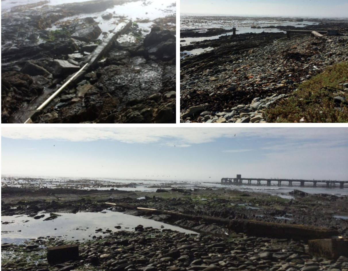
Figure 27: Some of the old sewage discharge pipelines discharging into the intertidal area on the eastern shore of Robben Island.
