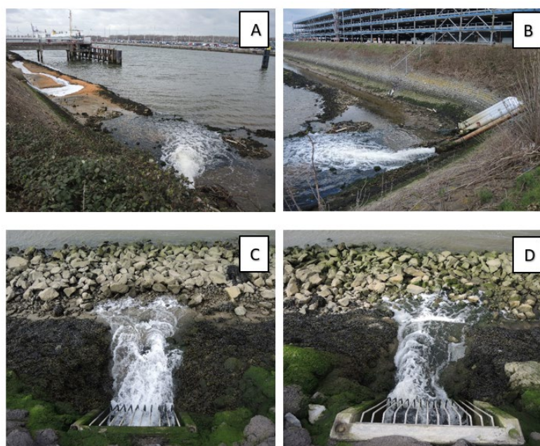
Figure 4 Brine discharge points (A: Discharge point of DWP Botlek on the right and discharge point of another industrial facility on the left in Brittaniëhaven area, B: Discharge point of DWP Botlek in Brittaniëhaven area, C & D: two discharge points of DWP Maasvlakte in Hartelkanaal area)
